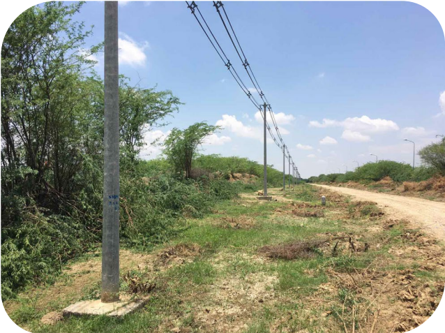
6.6kV Overhead Transmission Line
