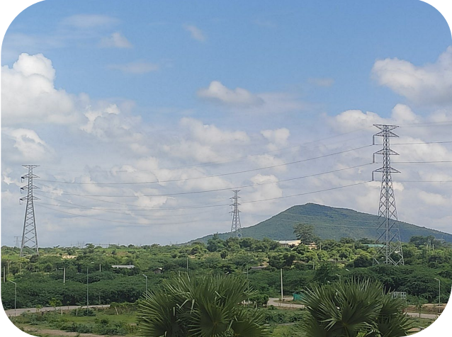
230 kV Transmission Tower
